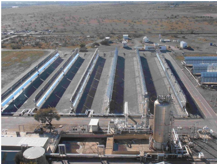
Figure 1 – An arial view of the collection lines of the TCP-100 facility
